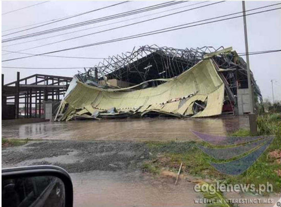
One of the many damaged buildings in Santiago, Isabela after the onslaught of typhoon Rosita (Yutu) (Eagle News Service)
